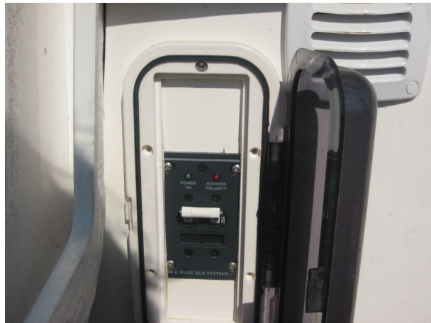
FIGURE 40 – SHORE POWER BREAKER IN COCKPIT
