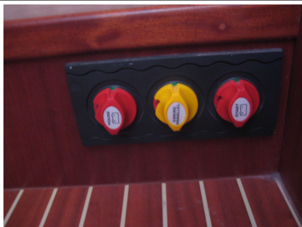
FIGURE 37 – BATTERY MASTER SWITCHES IN AFT BERTH
