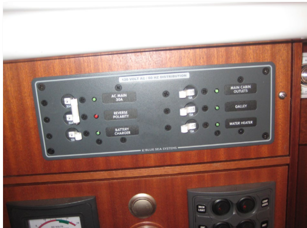
FIGURE 39 – MAIN AC PANEL BOARD IN SALON
