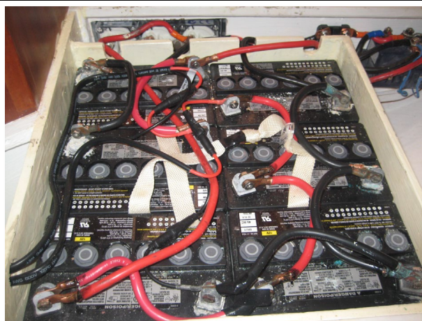
FIGURE 38 – ENGINE AND HOUSE BATTERIES
