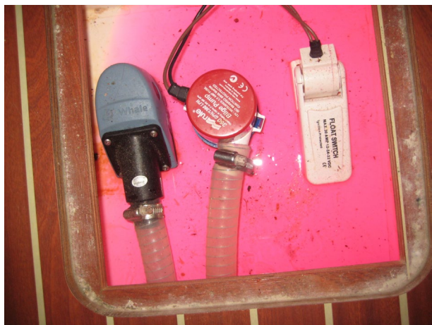
FIGURE 33 – BILGE PUMPS FITTED BELOW CABIN SOLE
