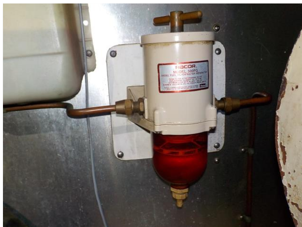
FIGURE 19 – FUEL FILTER IN ENGINE SPACE
