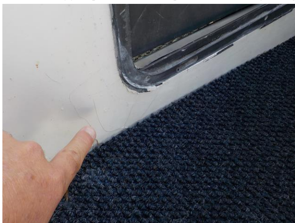
FIGURE 51 – DETERIORATED AREA AROUND SIDE DECK ACCESS DOORS
