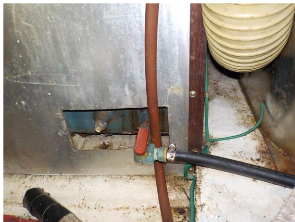
FIGURE 20 – TANK ENCLOSURE WITH BALL VALVE
