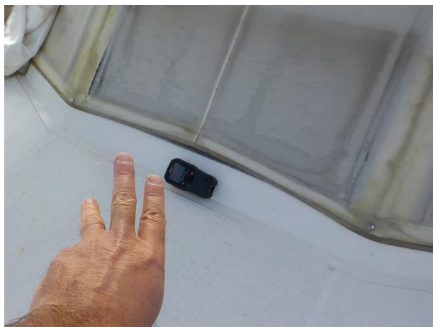
FIGURE 53 – ELEVATED MOISTURE IN FOREDECK
