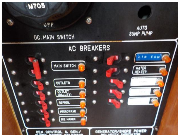
FIGURE 27 – MAIN AC PANEL BOARD IN SALON
