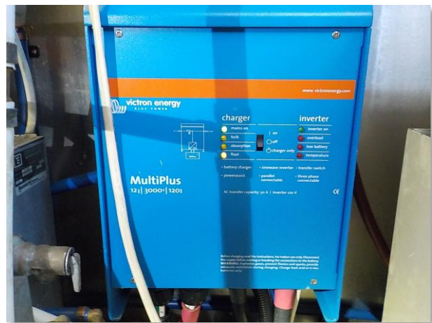
FIGURE 28 – CHARGER/INVERTER IN ENGINE SPACE
