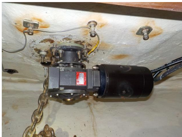
FIGURE 37 – WINDLASS IN FOREPEAK LOCKER
