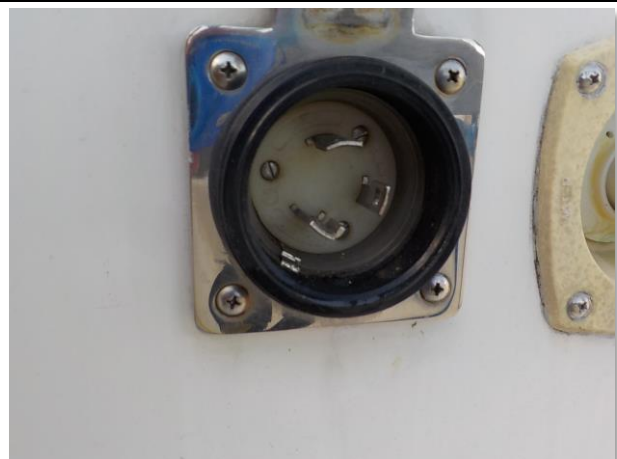
FIGURE 30 – SHORE POWER MAIN INLET RECEPTACLE
