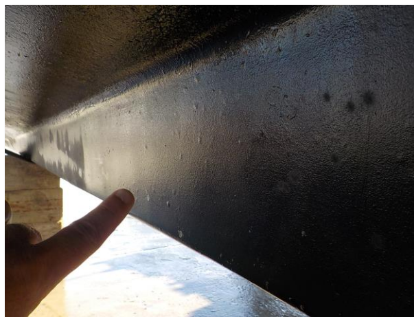
FIGURE 54 – NON-STRUCTURAL BLISTERS ON KEEL
