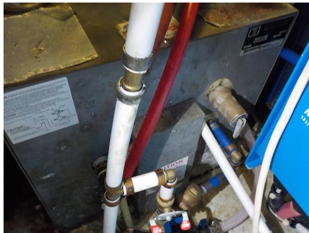
FIGURE 22 – HOT WATER TANK IN ENGINE SPACE
