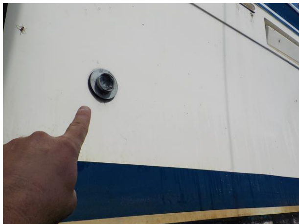
FIGURE 55 – SILICONE FILLED THROUGH-HULL STARBOARD TOPSIDES
