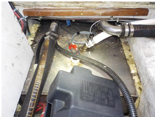
FIGURE 23 – HOLDING TANK IN ENGINE SPACE
