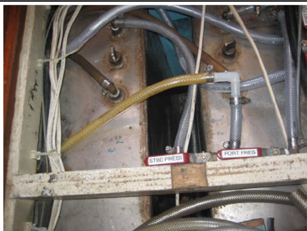
FIGURE 27 - FRESH WATER TANKS
