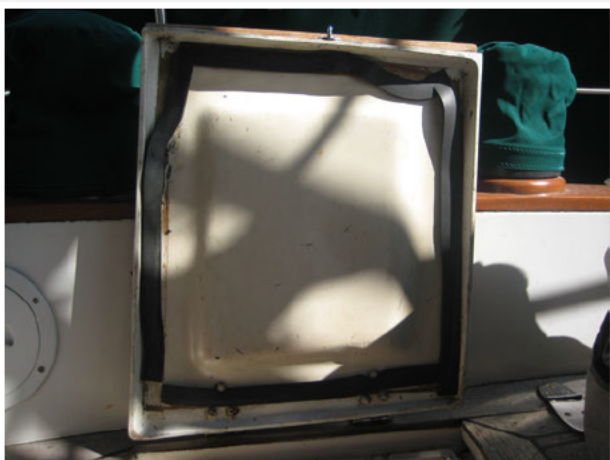
FIGURE 55 – LOOSE SEAL ON PROPANE LOCKER LID
