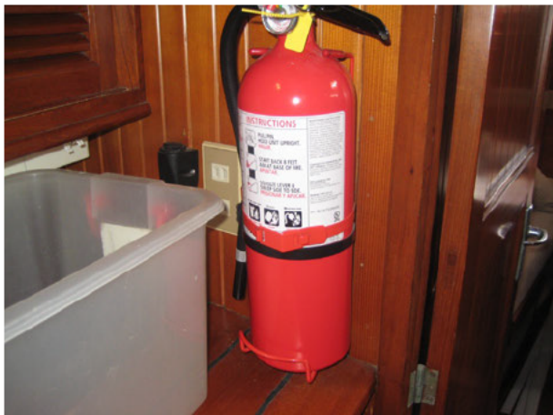
FIGURE 49 - PORTABLE FIRE EXTINGUISHER IN V-BERTH
