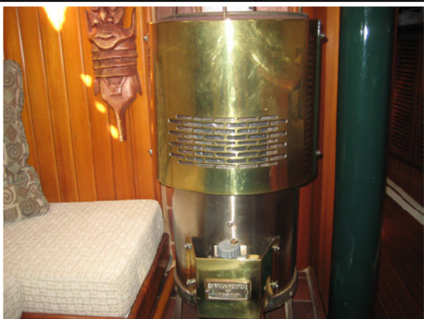
FIGURE 43 – DIESEL HEATER IN SALON
