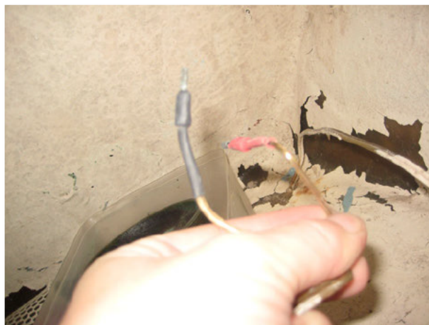
FIGURE 54 – BARE WIRE ENDS IN INSPECTION PORT AFT COCKPIT
