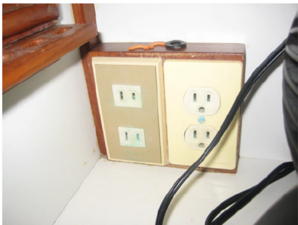
FIGURE 53 – NON-GFCI RECEPTACLES IN HEAD
