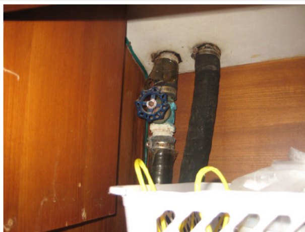
FIGURE 56 – CORROSION AT GATE VALVE IN WASTE PUMP OUT HOSE
