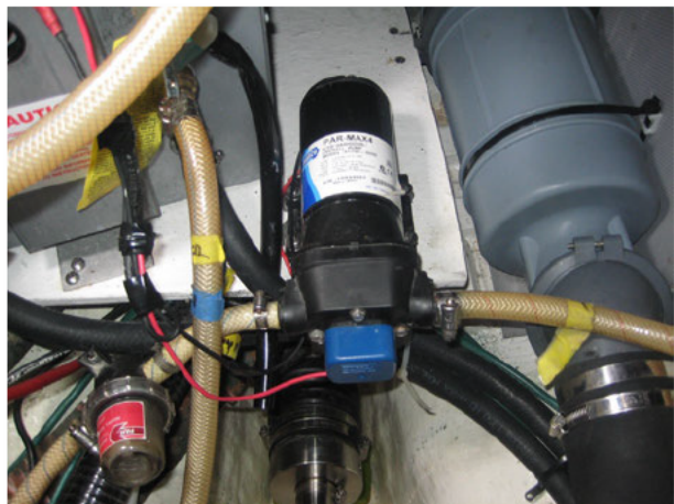
FIGURE 31 – AFT WASHDOWN PUMP
