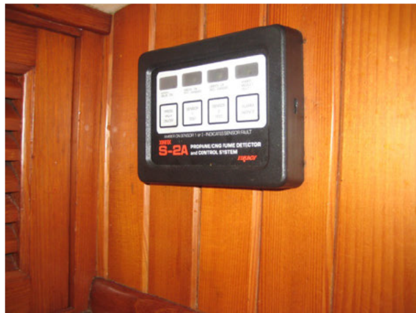
FIGURE 50 - PROPANE FUME DETECTOR IN GALLEY
