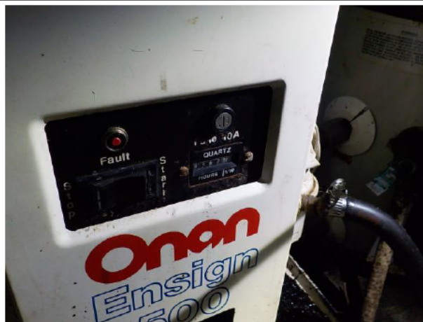
FIGURE 28 - HOUR METER FOR GENERATOR
