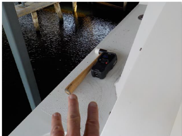
FIGURE 37 – ELEVATED MOISTURE OBSERVED PORT SIDE LOWER SIDE DECK
