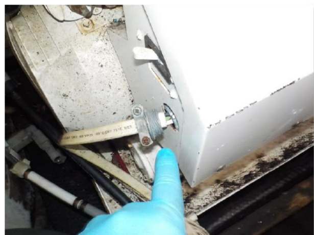
FIGURE 36 – UNSUPPORTED WIRE OBSERVED ON GENERATOR ENCLOSURE IN THE ENGINE SPACE
