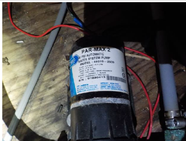
FIGURE 20 - WATER SYSTEM PUMP
