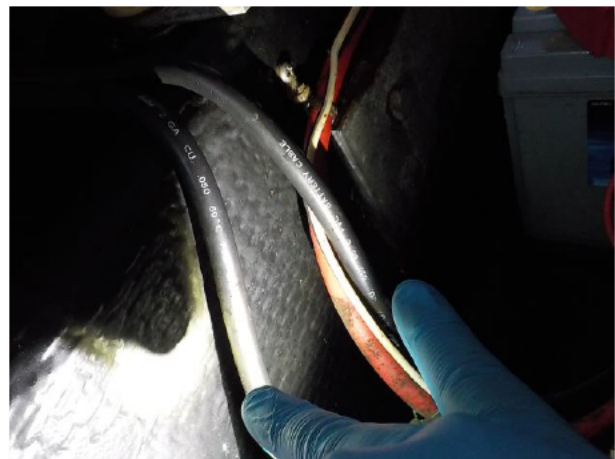
FIGURE 34 – NON-APPROVED WIRE TYPE OBSERVED AT BATTERY CABLES IN THE ENGINE SPACE
