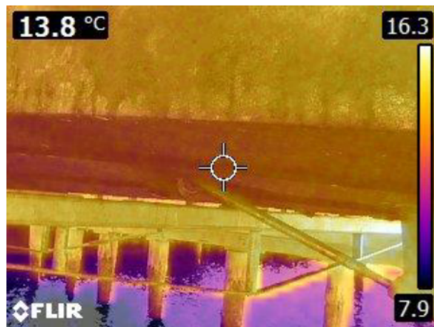
FIGURE 2 - THERMAL IMAGE OF TRANSOM
