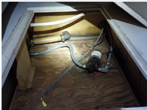
FIGURE 19 - WATER TANK AND PUMP BELOW AFT BERTH
